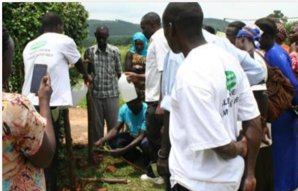
VHTs constructing a tippy tap at St James Health Center III in Masiriba Village
